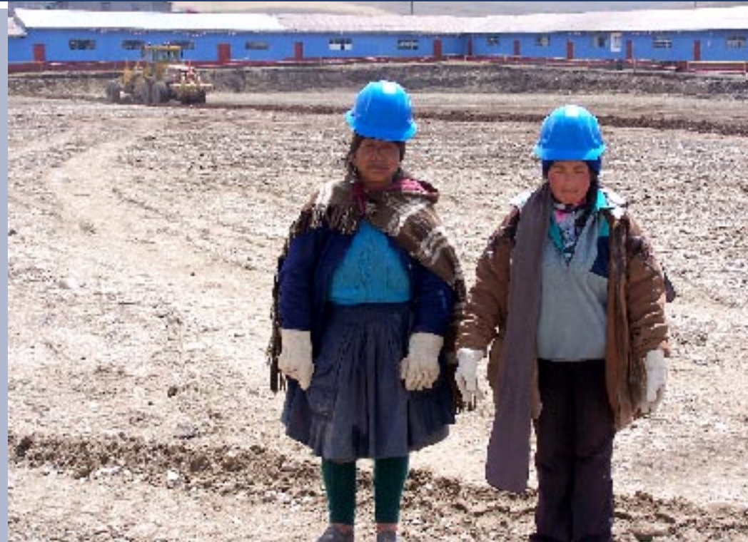
VALUING OUR LOCAL COMMUNITIES: TWO HARD- WORKING LOCAL WOMEN EMPLOYED CONSTRUCTING THE ROCK RETAINING WALL, HARDHATS SECURE OVER THEIR TRADITIONAL HEAD-WEAR
