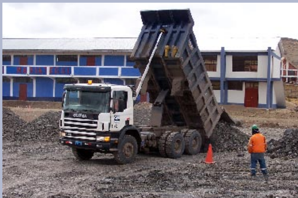
SCANIA TIP-TRUCK BRINGING IN WASTE MATERIAL FROM THE PIT FOR THE BULK FILL
